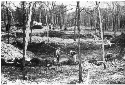
Figure 11. Digging foundations while saving trees at Wildwood Park during construction in 1947. (Photo used with permission of Wildwood Park History Book Committee.)
