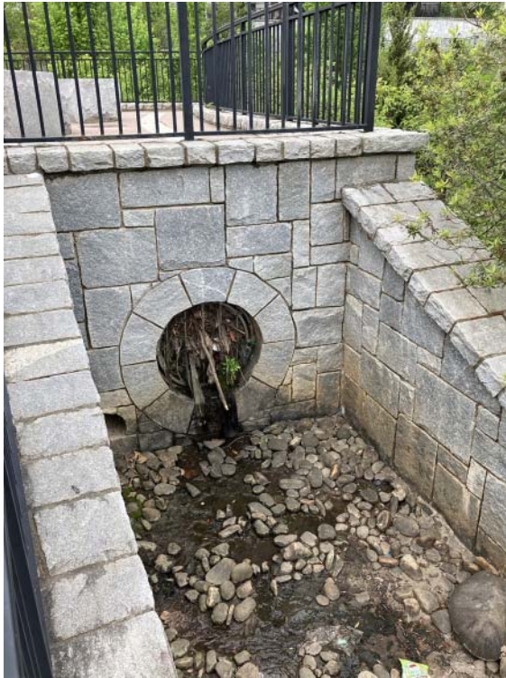
Figure 12 A pipe outlet carrying rainwater at Historic Fourth Ward Park is blocked by debris, potentially diminishing visitor appreciation for the rain message. Design: HDR; photograph: Eliza Pennypacker, 2021.
